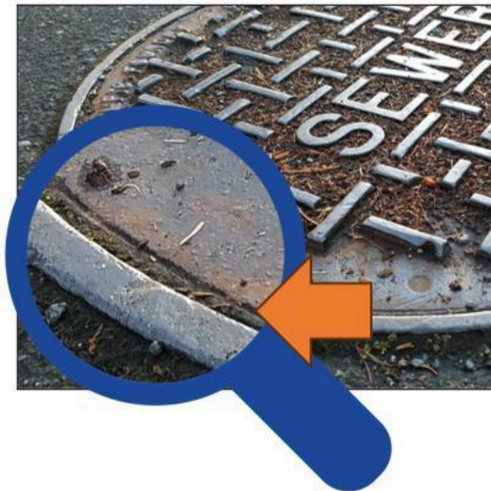
Close up of debris that may make manhole cover removal difficult
